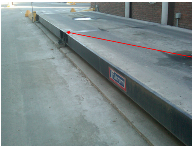
Weighbridge Modules bolted together forming a singular rigid fixed structure
