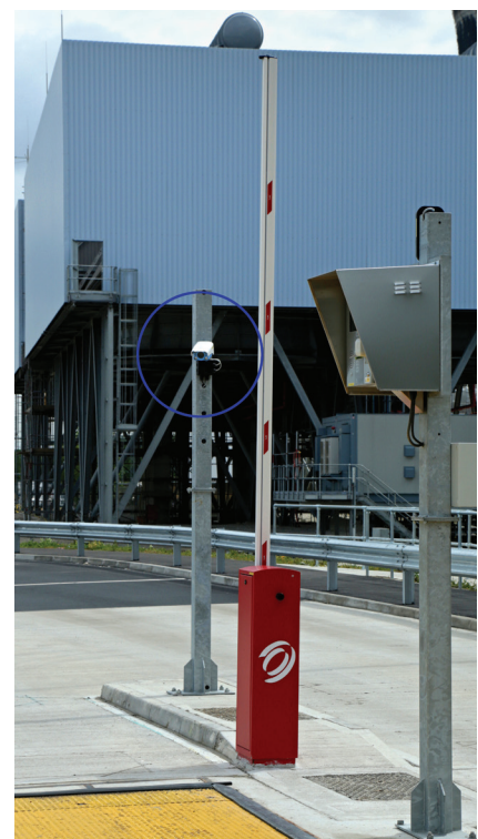
ANPR camera (circled) and driver terminal
